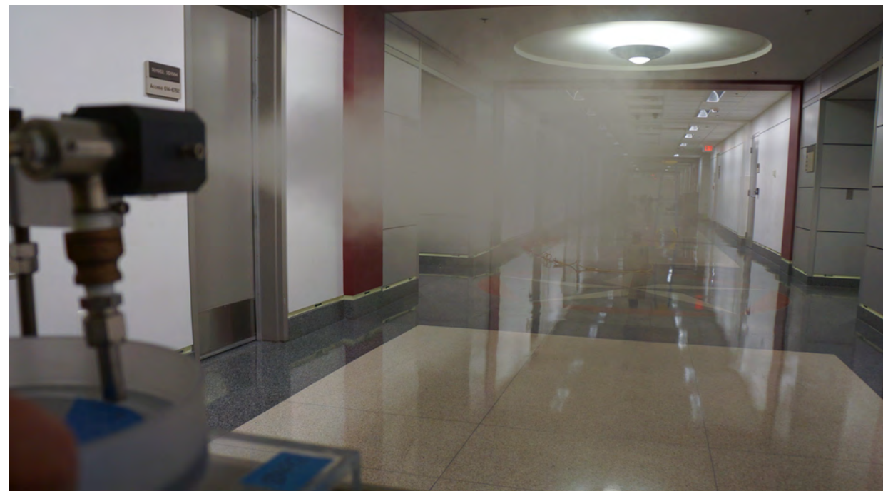
In coordination with the Pentagon Force Protection Agency, researchers released DNATrax microparticles—multiple types of particles with unique DNA barcodes—to reveal air circulation or stagnation resulting from the Pentagon's heating, ventilation, and air conditioning systems.
