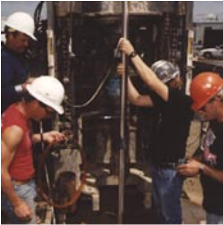
(E&TR July 1992) Effective, rapid removal of underground hydrocarbon spills can be done with dynamic underground stripping. Workers are drilling a steam injection and electrical heating test well that will be used for controlled extraction of contaminants and associated groundwater from spills such as a leaking diesel fuel tank.
