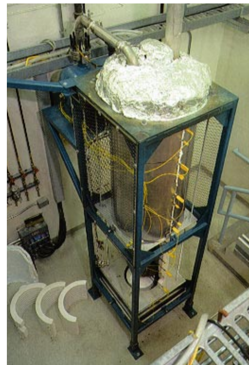
A view of the molten salt crucible and associated piping from above. The slurry of waste and air enters the top of the crucible, and off-gases exit through the larger pipe on the right.
