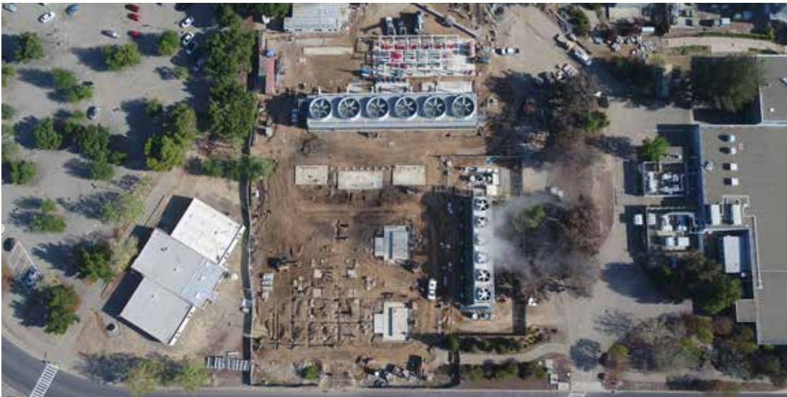
A little more than a year into construction, the new cooling towers and pump system had been built, and work to install the electrical substation progressed.
