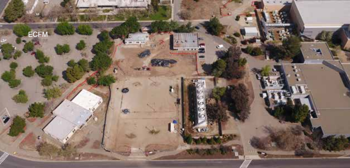
In March 2020, the site for the substation and cooling towers serving the Exascale Computing Facility had only just been cleared and prepared for construction.
